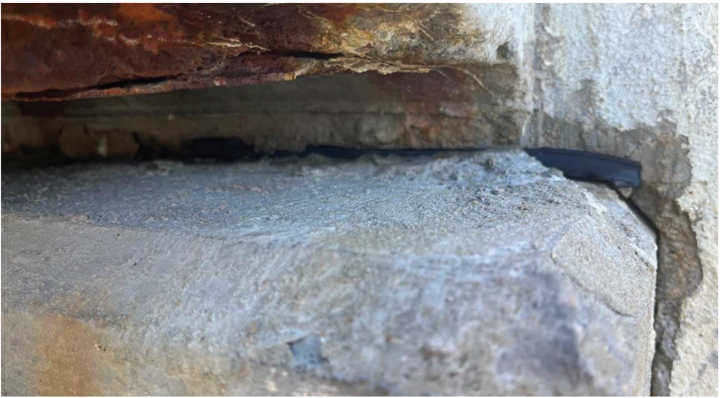
PHOTO # 5 View of rubber vibration dampener between pier cap and decking, not suspect.
