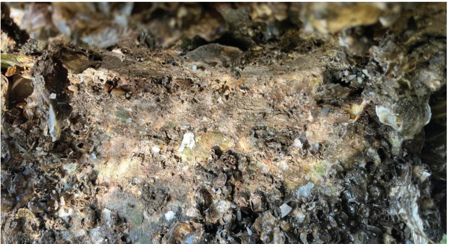
PHOTO # 6 View in between pier and pier cap, no material was able to be recovered from the joint.
