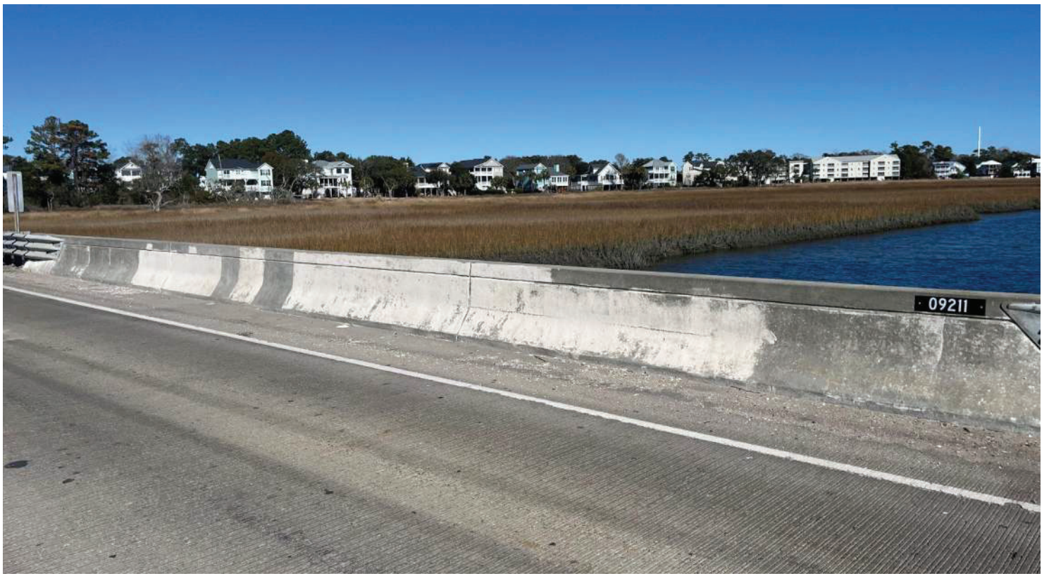
PHOTO # 7 View of HA #1 and LP-3, material was sampled for both lead and asbestos.
